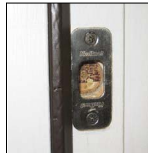
Photo 2B Dust plug has been removed
